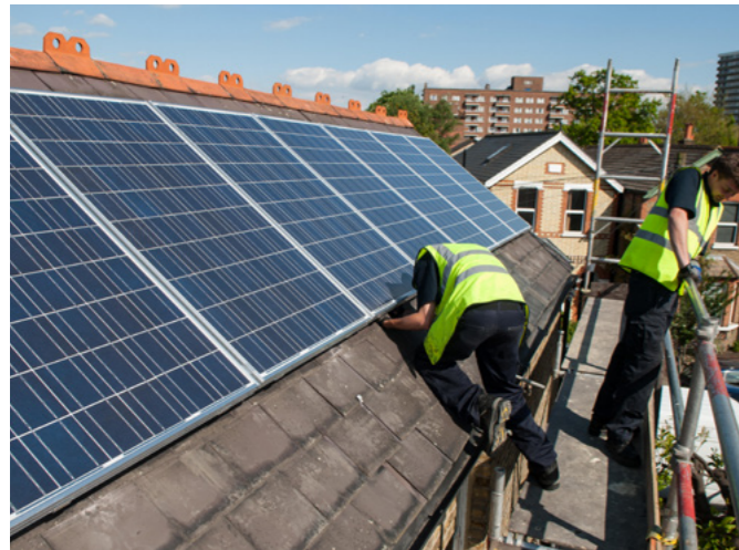
Figure 11 Solar Panel installations
